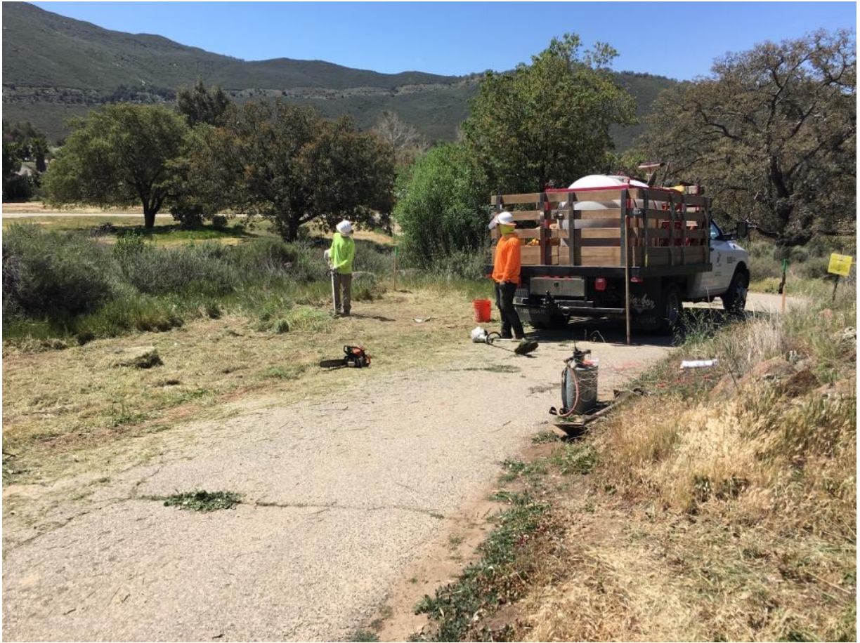
Photo 5: A crew is observed removing vegetation at Pole Z118074 (TL 682). Fire tools were observed within 50 feet of activity in accordance with the Construction Fire Protection and Prevention Plan (MM FF-1). Native American and biological monitors were present to observe vegetation clearing and removal in accordance with MM BIO-3, APM CUL-04, and the HPMP.
