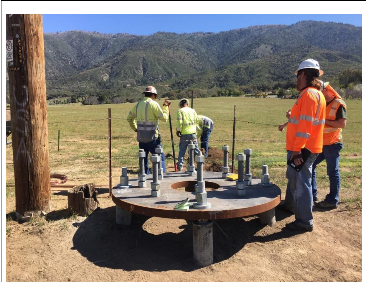
Photo 3: A crew digs a trench with hand tools to install grounding rods at pole Z118035 (TL 682) with biological and archaeological monitors present, in accordance with MM BIO-3, MM CUL-1, and APM CUL-04.
