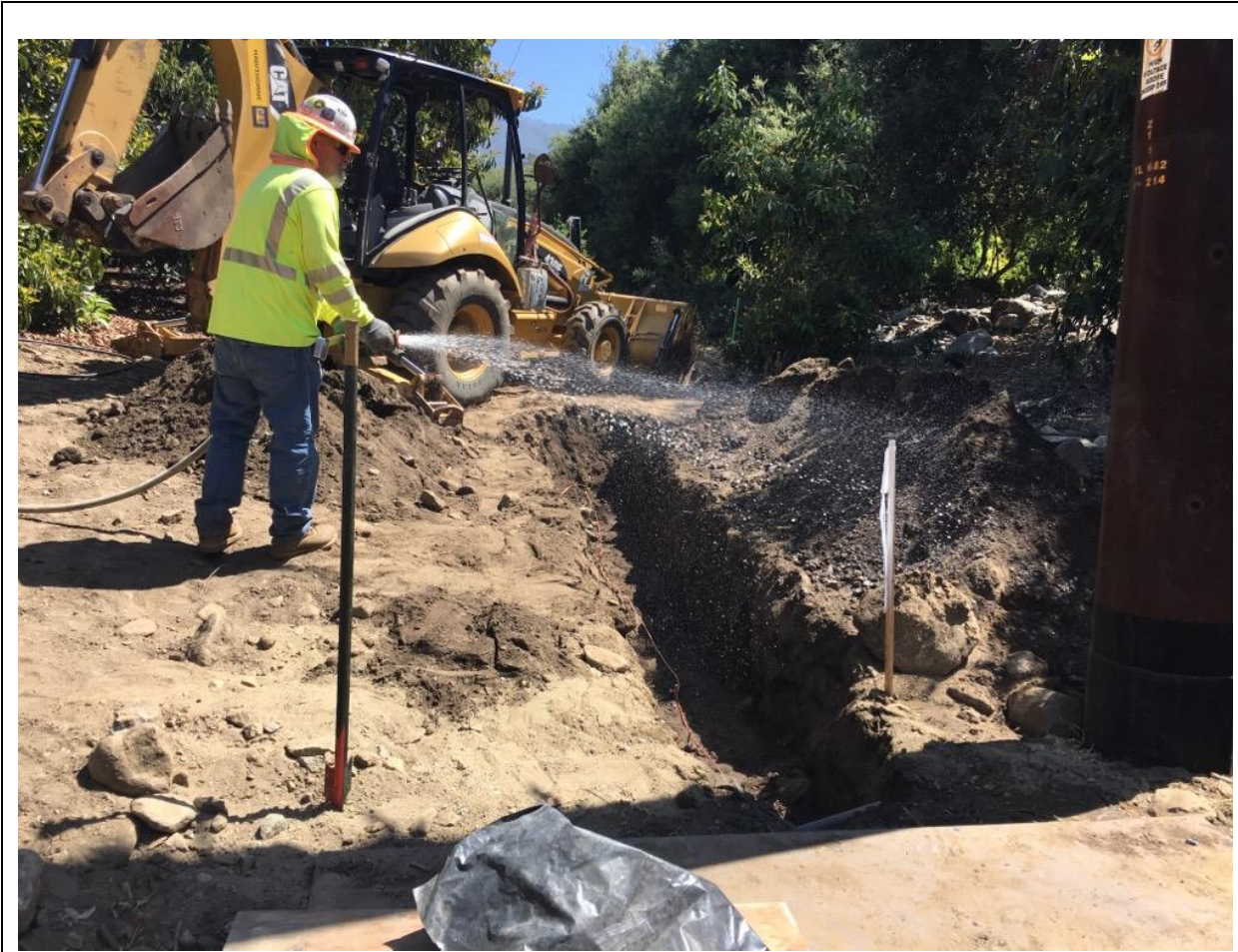
Photo 2: During grounding rod installation at TL 682, a crew member waters down spoils before backfilling in order to reduce fugitive dust emissions in accordance with APM AIR-02.
