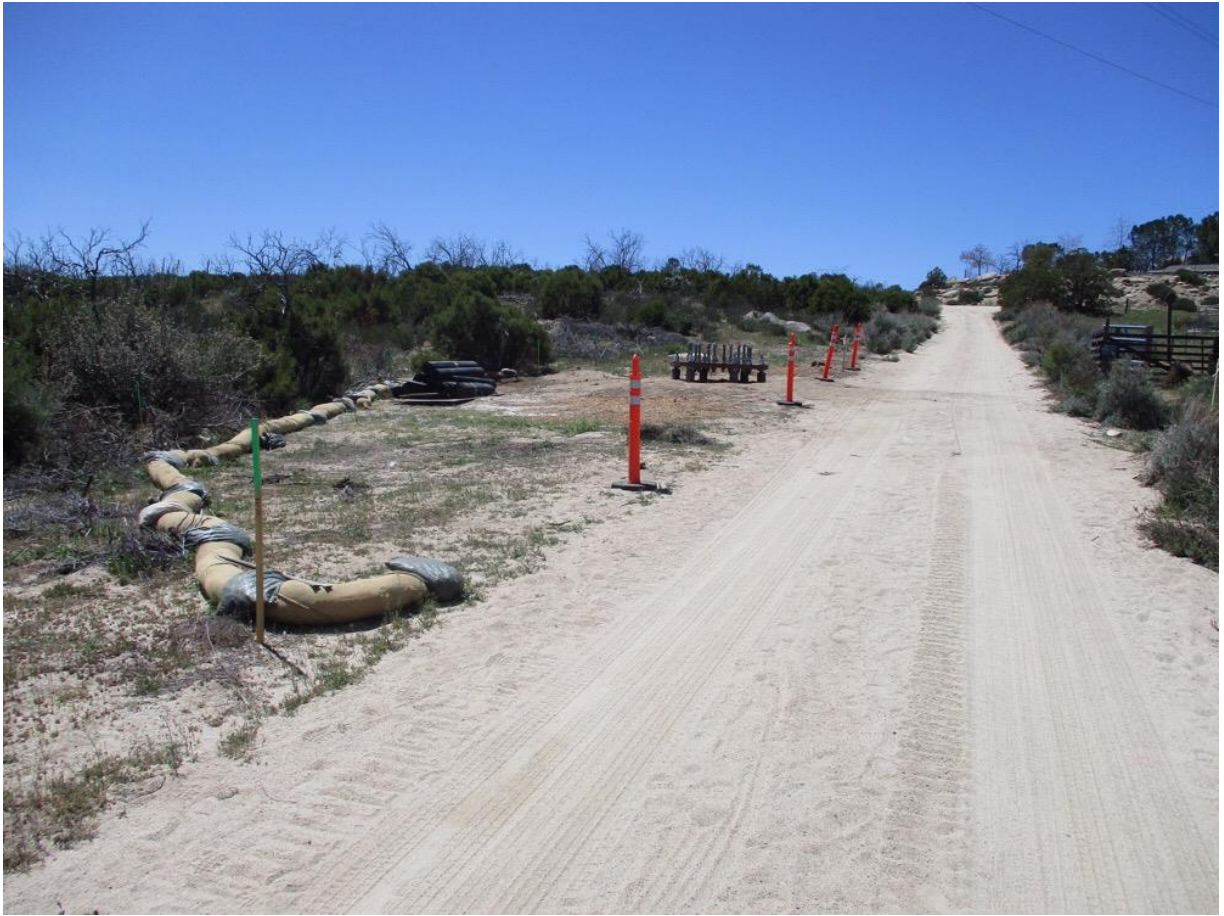
Photo 6: At Z44226 (TL 629E), perimeter fiber rolls were observed installed in accordance with the Erosion Control Plan and SWPPP.
