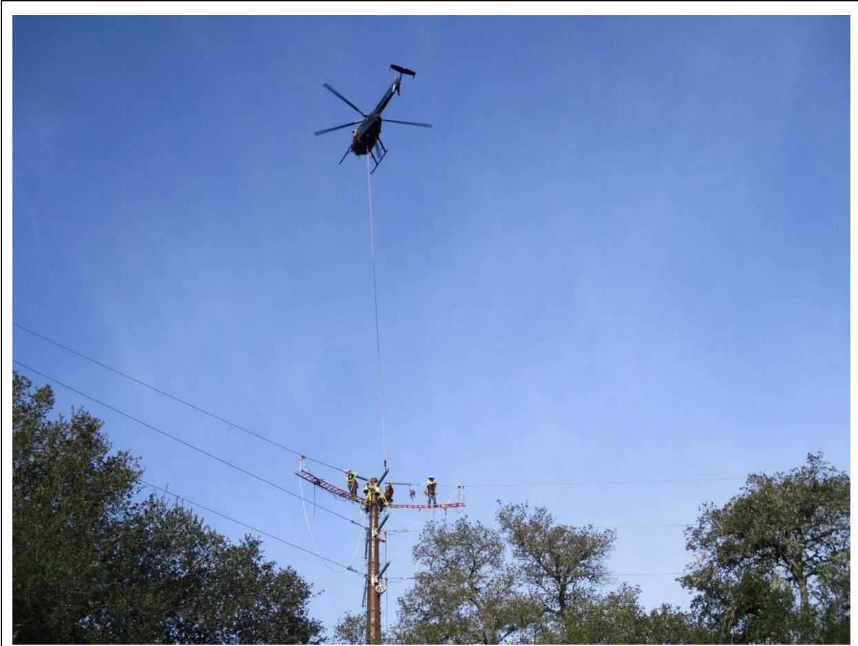
Photo 1: A crew is observed dead-ending transmission lines at Z118145 (TL 682). A helicopter was used to transport linemen to the tower using human external cargo operations in accordance with the Aviation Safety Plan and MM PHS-5.
