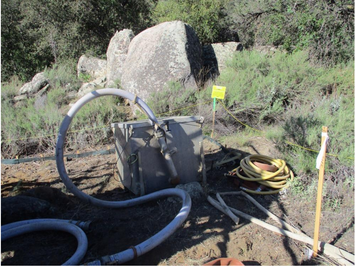
Photo 4: During drill site setup at a pole site along TL 682, a cultural ESA fence was observed installed around the perimeter of the workspace by the archeological monitor, in accordance with the HPMP and MM CUL-1. A containment box was staged on site to catch drill cuttings and reduce dust emissions in accordance with APM AIR-02.
